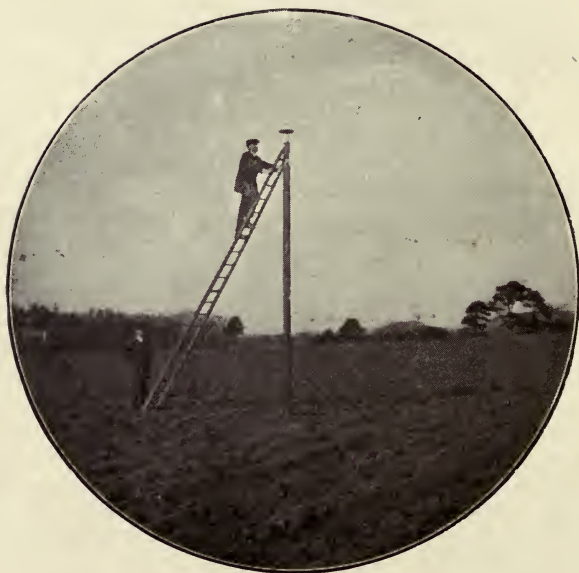
Placing an insulator upon one of the poles to carry electric discharge wire. The pole is fifteen feet high and the top portion of the insulator is about ten inches in diameter.
